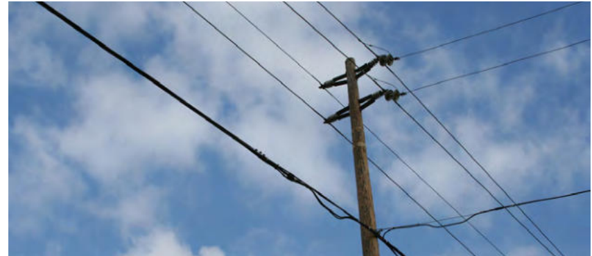
EXISTING TRANSMISSION LINE
